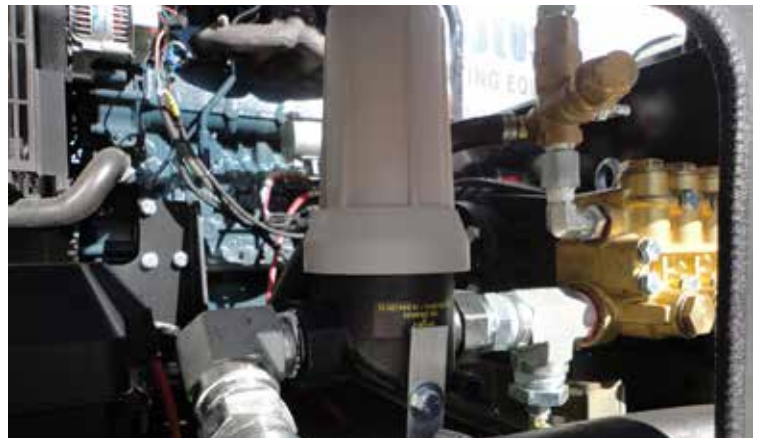
Pre-Pump Water Filters & Safety Bypass Valves
